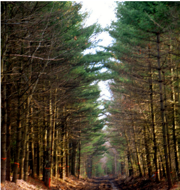
The trail under construction in Westford at Rt. 27/225 looking north Photo by Emily Teller– April 2008
