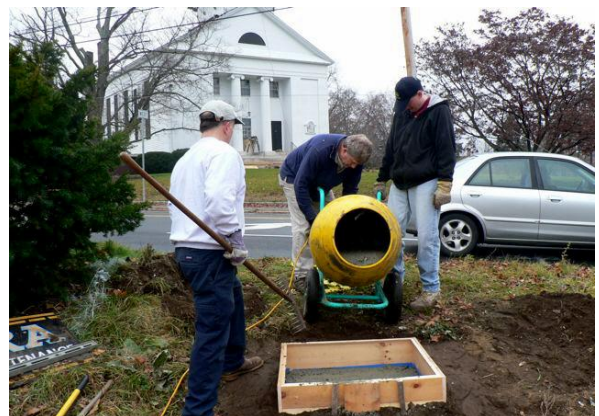
Tom Gazda, Ken Dews, and Mike Koziel pouring concrete for the Station Master base
